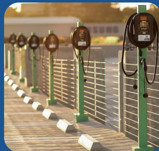
PowerFlex EV charging technology shown at a representative location
